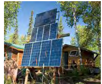
Solar panels in Kanuti National Wildlife Refuge. Image: Steve Hillebrand, USFWS.
