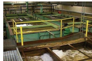
Aeration Chamber & Filter Trains at the Water Treatment Plant
