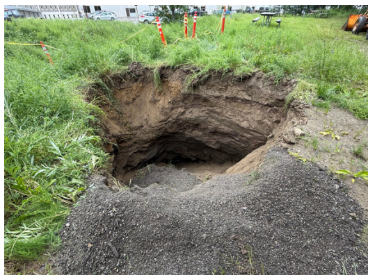
A new sinkhole opened up north of O'Neill on July 15, measuring about 20 feet across and 27 feet deep. Thanks to Raif and Jamie from the Grounds Crew for quickly and safely collapsing the hole and filling it in. photo by N. Platt
