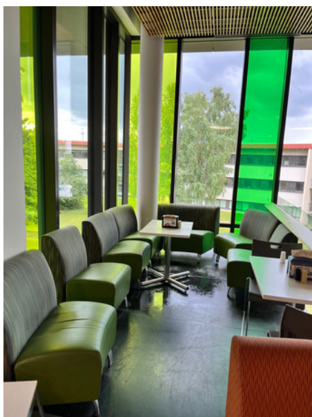
Wood Center Dining: We always get excited about a new roof leak. This one happened during an epic rainstorm on July 13. A loose roof drain collar caused this puddle. Thanks to James in the carpentry shop, it's been repaired. photo by N. Platt
