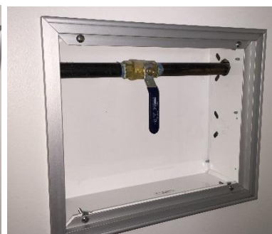
Figure 4. Valve handle in "off" position
