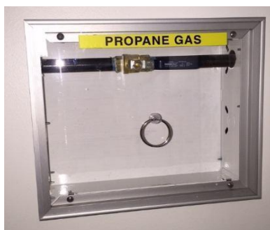
Figure 2. Propane gas shut-off valve
