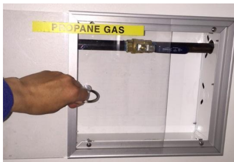
Figure 3. Removal of Plexiglass plate covering valve
