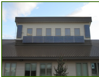
Solar Panels at UAF Bristol Bay Campus.
