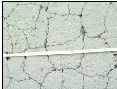
Fatigue Cracking in Polymer-modified asphalt mix; photo courtesy of AKDOT&PF.
