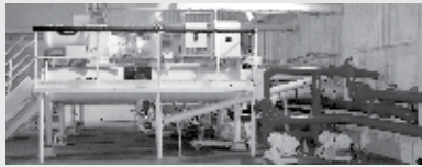
Organic Rankine Cycle (ORC) Geothermal Power Plant
