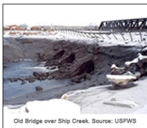
Figure 20: Collapsing culverts at mouth of Lower Ship Creek, 2002.
