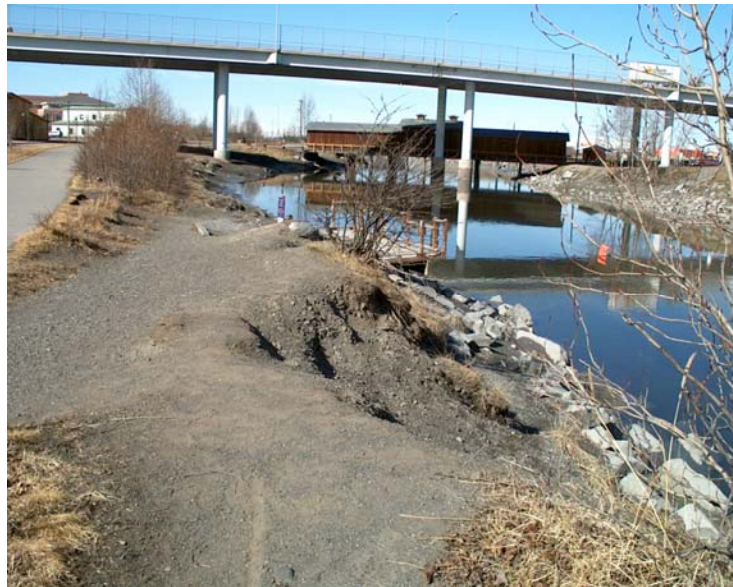
Figure 14: Bank Erosion, Ship Creek, 2003.
