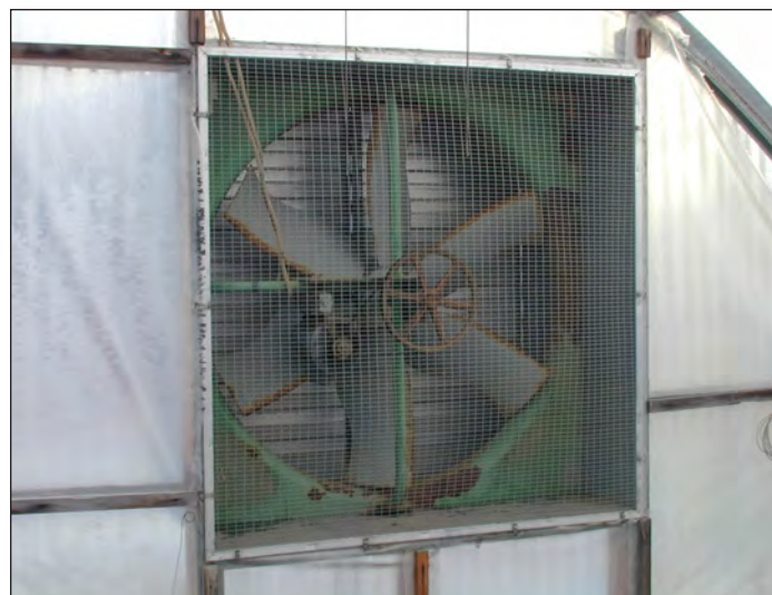
Picture 5. A multi-speed fan helps regulate greenhouse temperature throughout the season.
