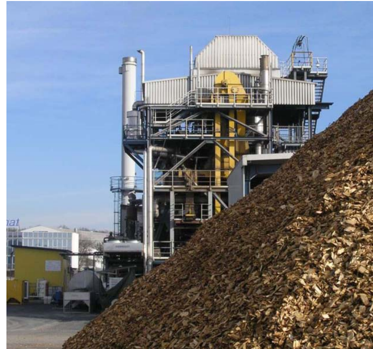
2 MW plant in Güssing, Austria
