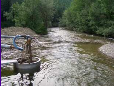
Monument Creek Provides Cooling Water (~40F)
