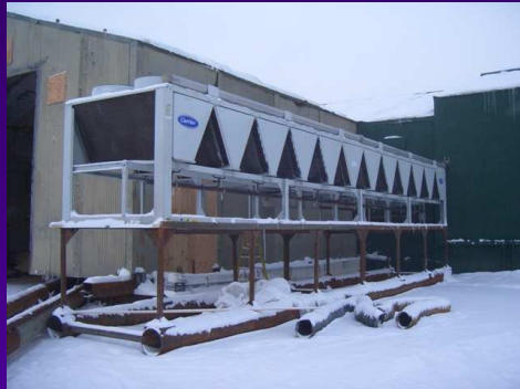
Air cooled condenser
