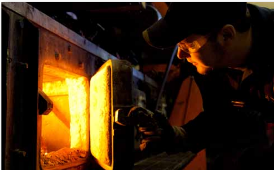
Maintenance technician Dean Ojala checks the flame in a coal-fired boiler at the UAF power plant, one of two such boilers that have been in use at UAF since the 1960s.
