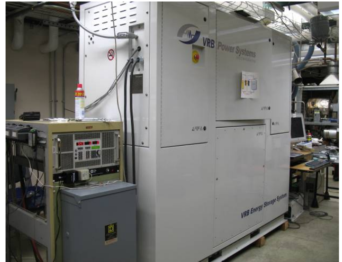
10kW VRB battery system currently undergoing testing at the University of Alaska
