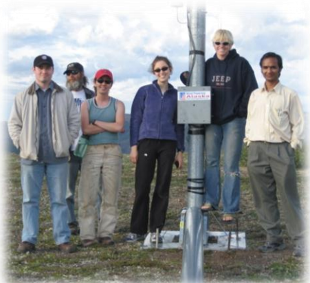
Installing a wind anemometer at Chena Hot Springs Resort. Photo by G. Holdmann, ACEP
